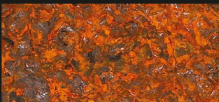
Without corrosion protection treatment
